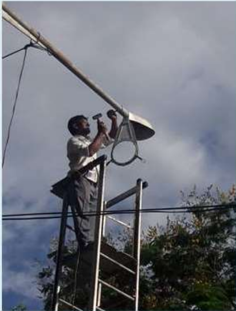
Work undertaken to replace conventional Electrical Bulbs and Tube lights with LEDs
