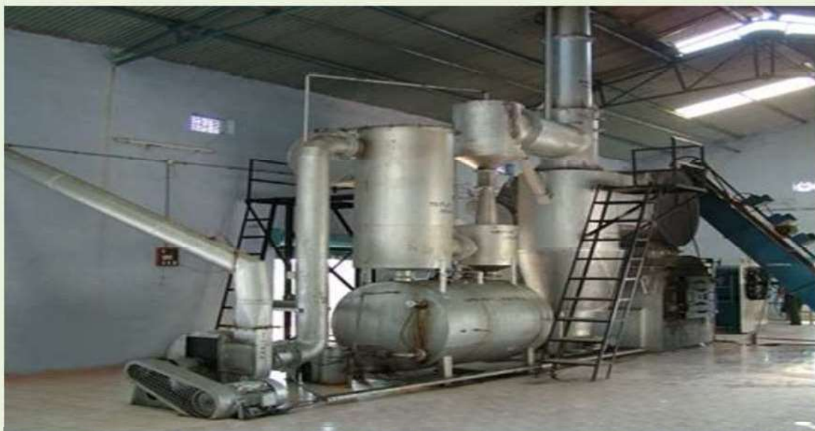
Kakatiya Toxic Waste Treatment Plant, Hanamkonda
